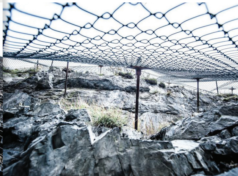
An example of a slope mesh system designed to protect a highway from falling ice that builds up on the slopes during the winter.
