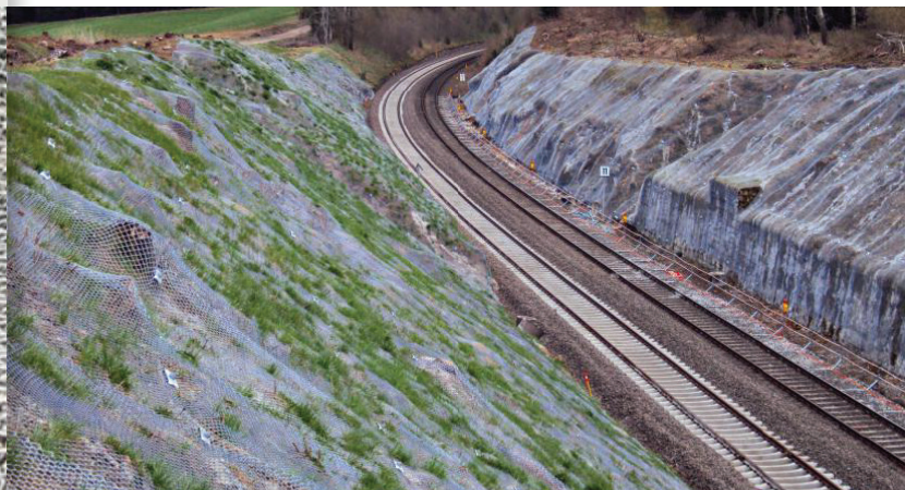
Railway cuts and existing walls stabilized using High Performance Netting.
