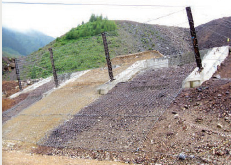
Before photo of a 3000 kJ hybrid test. The system consists of 5 m high posts with 12 m of Omega-Net.
