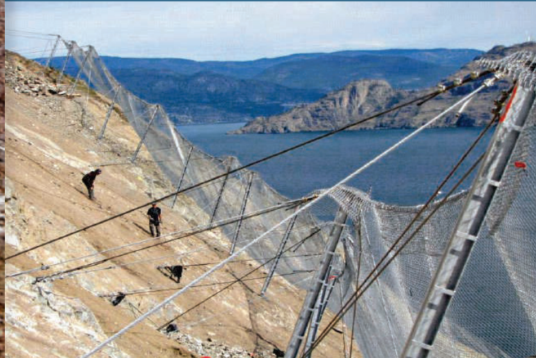
A lower energy attenuator system composed of High Performance Netting in combination with standard hinged posts and base plates.
